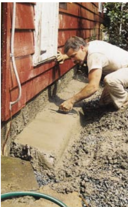
Figure 4. The stiff mix was easy to mold and trowel at the top of the foundation, where 6 inches of the new foundation remained visible.
