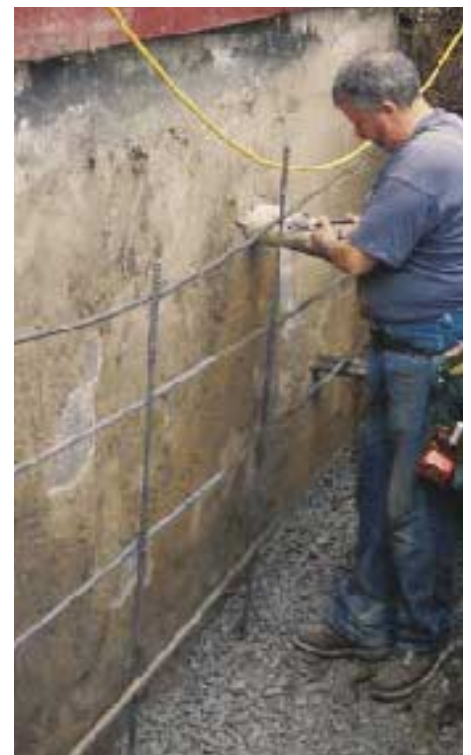
Figure 2. After the trench was dug, the author installed #5 rebar 4 feet on-center vertically, and 2 feet on-center horizontally.
