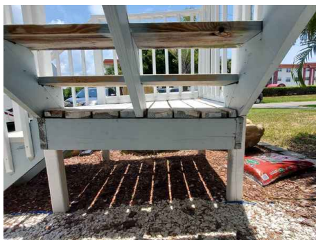
4. Settling/twisting of landing
