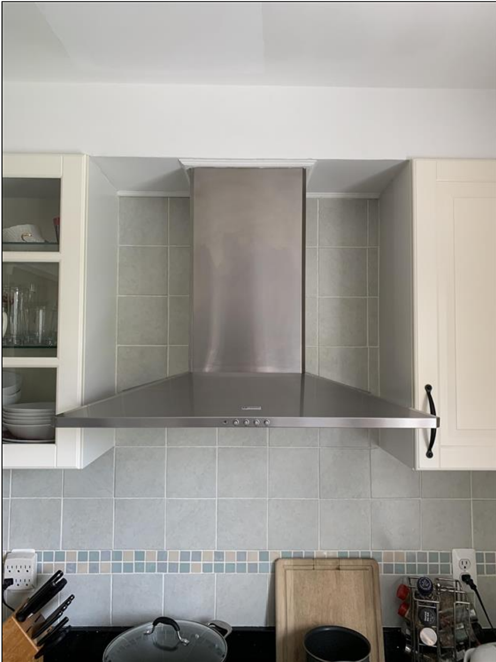
10.1 Item 3(Picture) Range hood on second floor.
