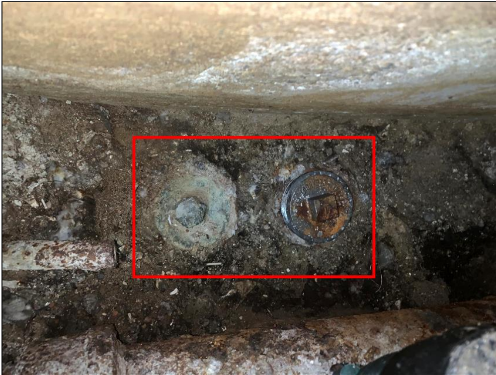
6.0 Item 2(Picture) Sewer trap. One of the caps is newer which may indicate the a repair or the removal of a clog.
