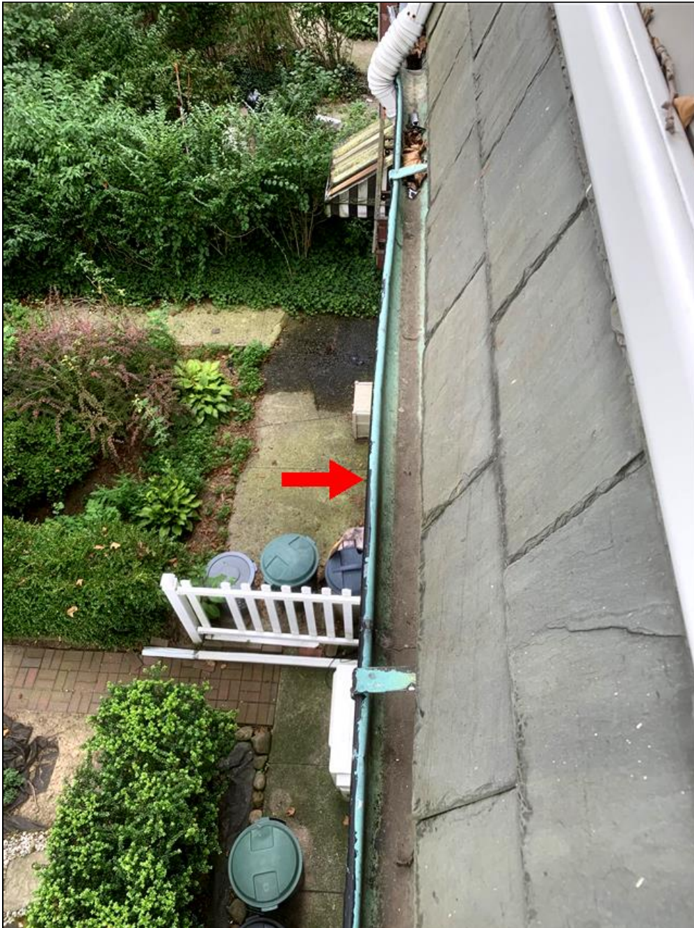
1.3 Item 3(Picture) Gutter serving slate roof at the font of the home.
