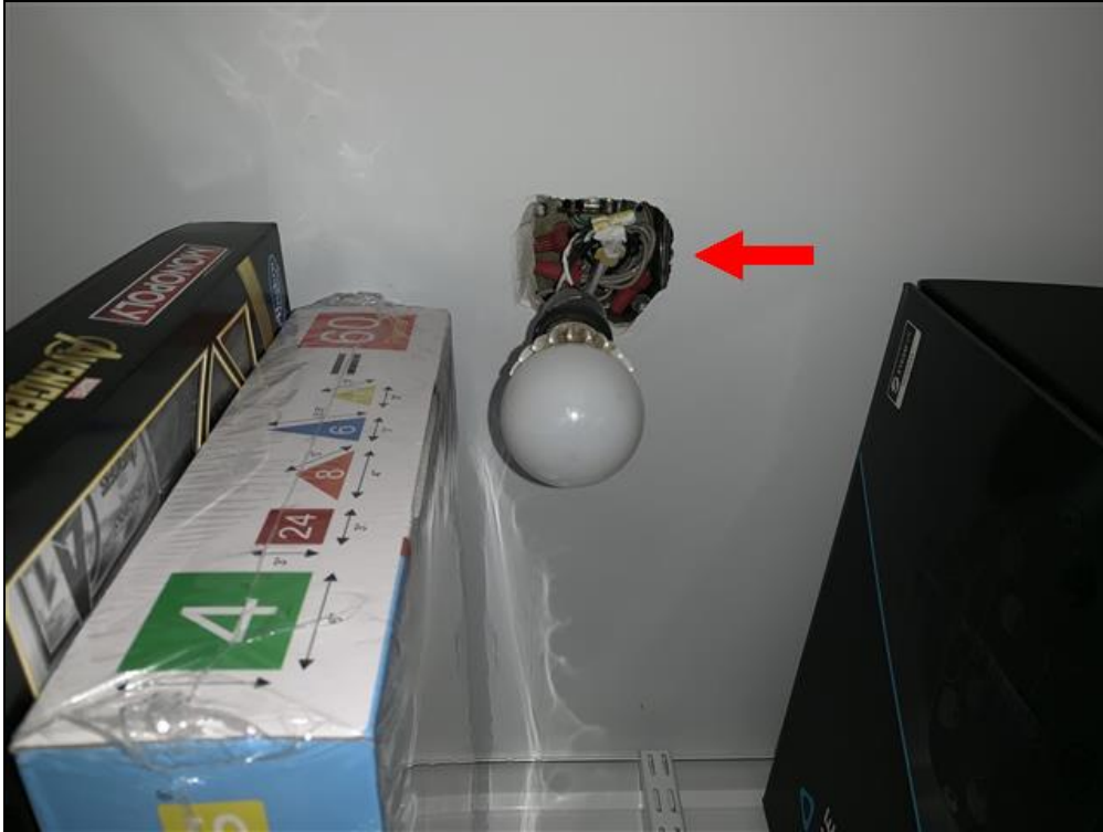
7.3 Item 3(Picture) Exposed wires in first floor bedroom closet.
