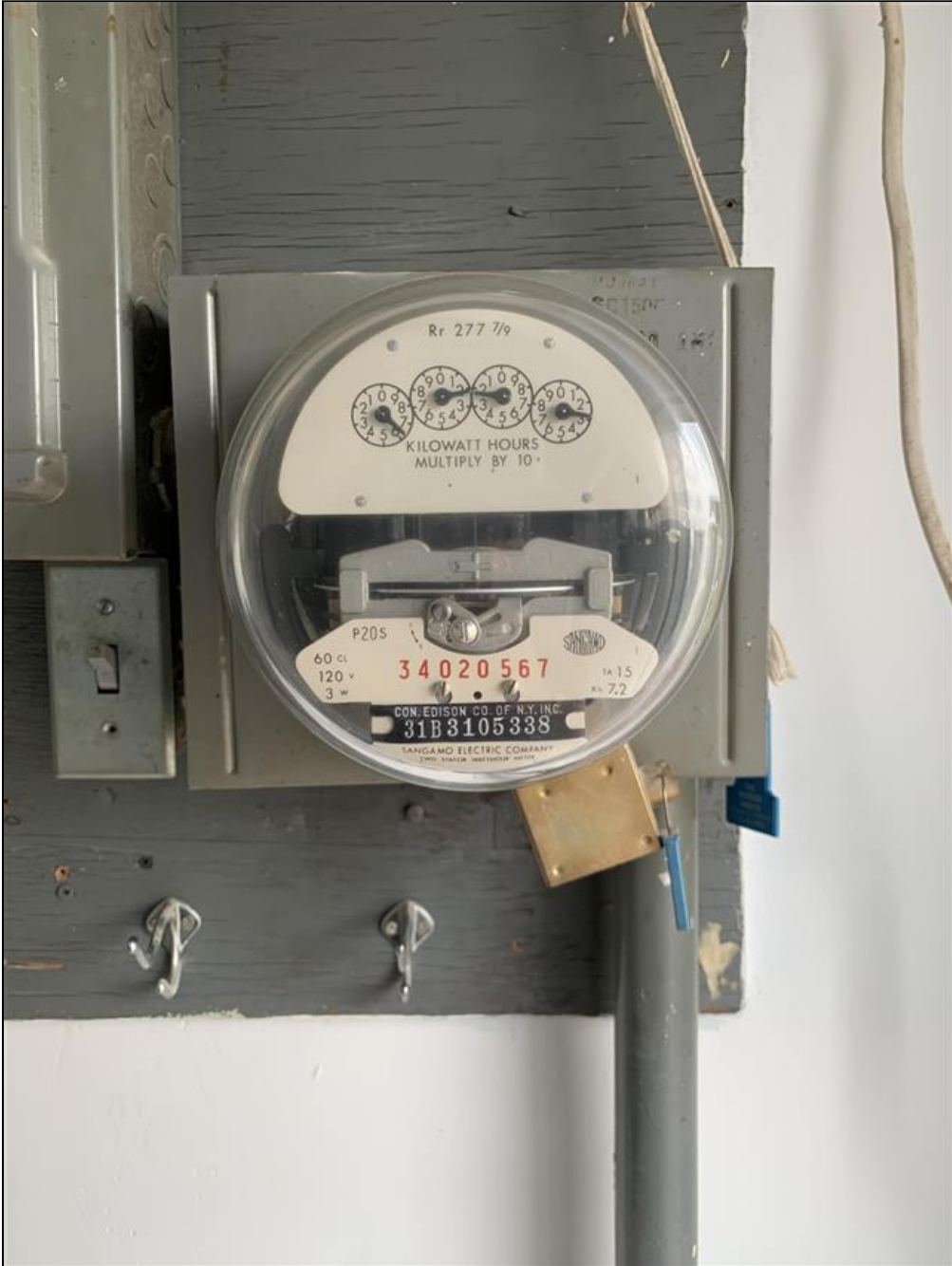
7.0 Item 2(Picture) Electrical meter.
