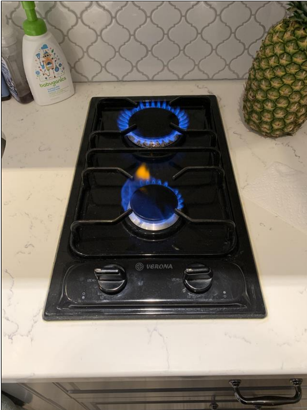
10.0 Item 1(Picture) Verona gas range on first floor.
