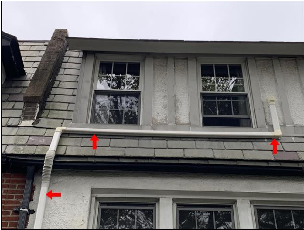
8.8 Item 4(Picture) Conduit for third floor HVAC condensation drainage.
