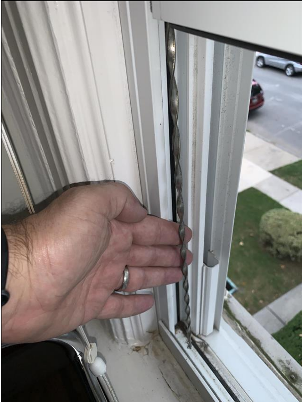
4.7 Item 2(Picture) A window channel balance was found to be disconnected or broken in the third floor walk-in-closet / bedroom.
