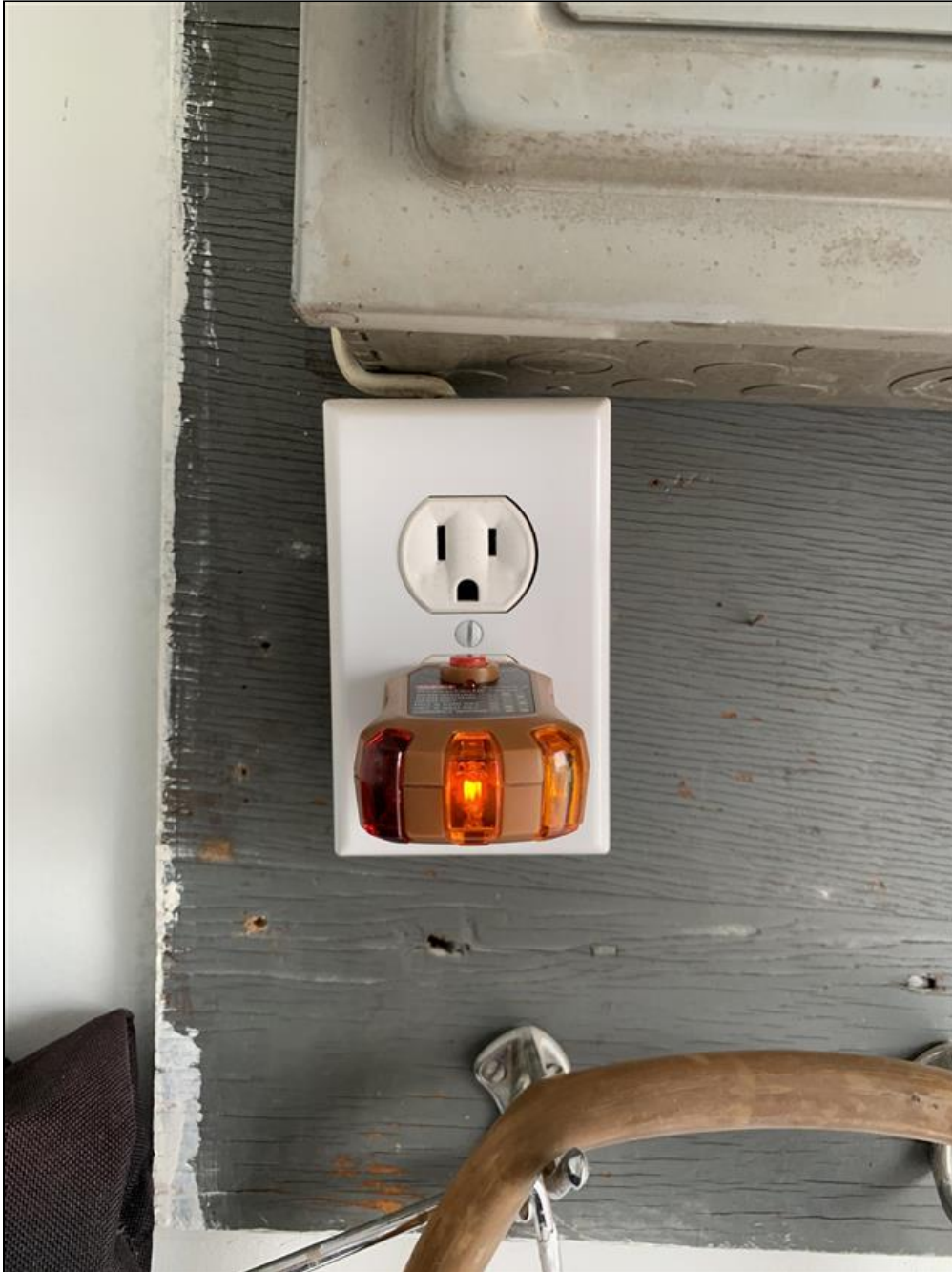
7.3 Item 5(Picture) Loose or missing ground.
