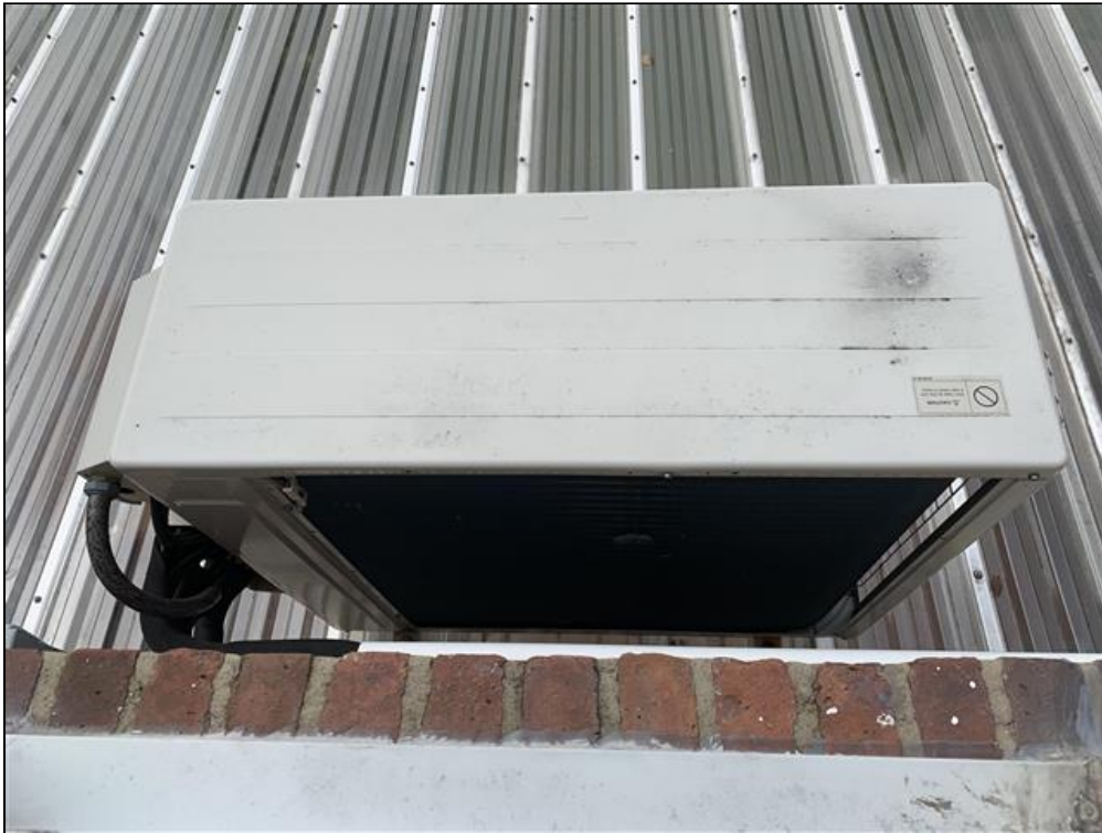
8.0 Item 3(Picture) Heat Pump mounted outside second floor kitchen window.
