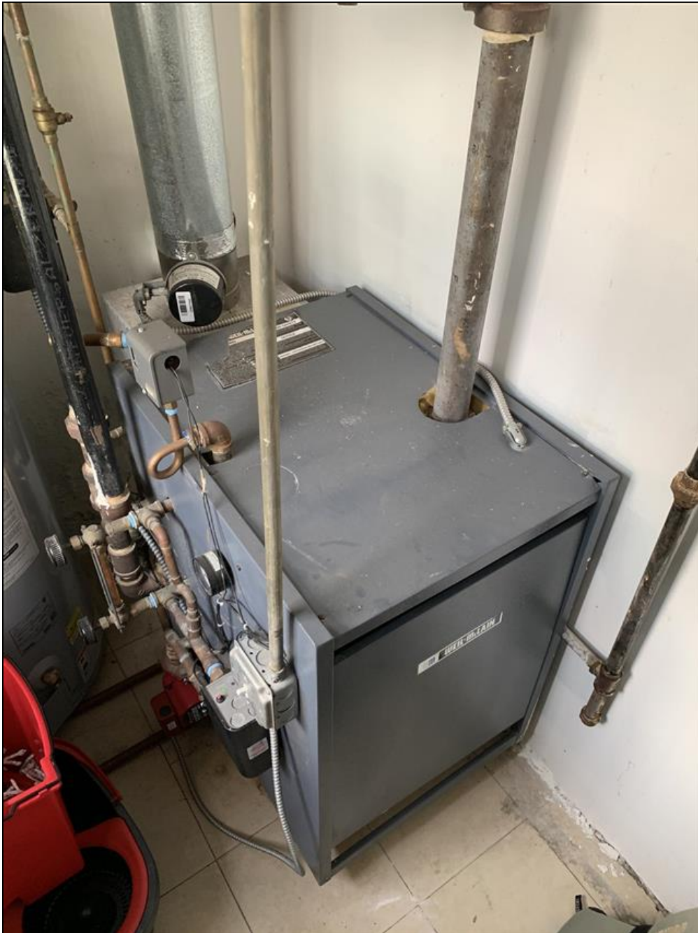
8.0 Item 1(Picture) Weil-McLain boiler.
