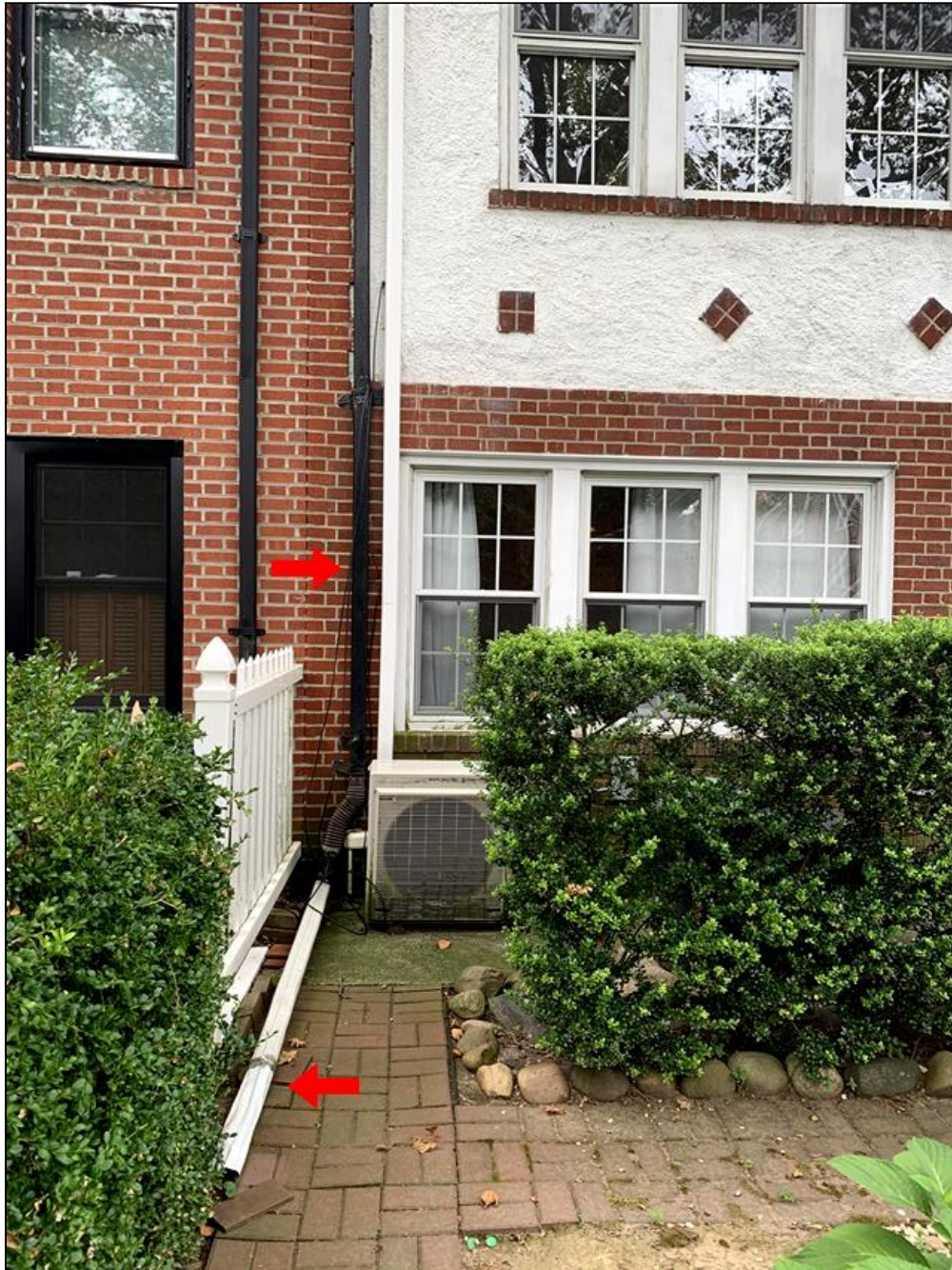
1.3 Item 5(Picture) Left-hand downspout terminates a good distance away from home.
