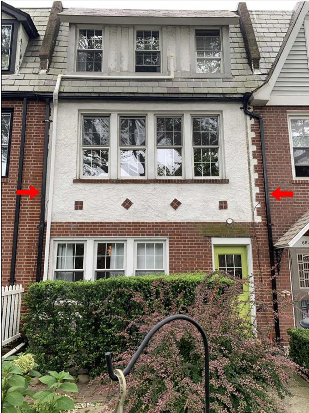
1.3 Item 4(Picture) Downspouts from gutter at front of home.
