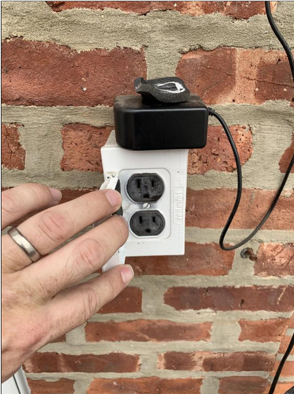
7.4 Item 1(Picture) Rear of home: Exterior electrical receptacles should be GFCI protected for added safety.
