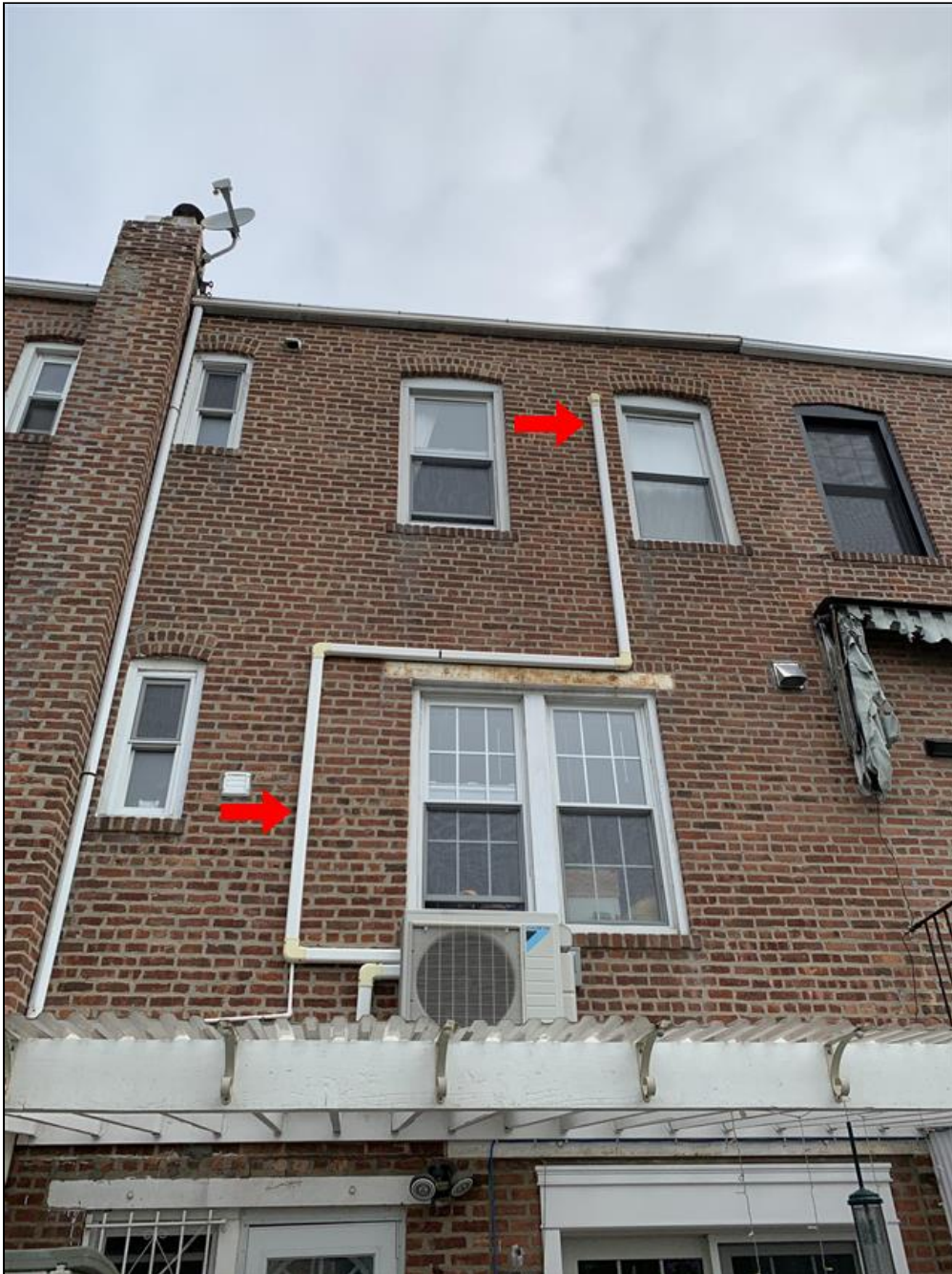
8.8 Item 5(Picture) Conduit for third floor HVAC condensation drainage.
