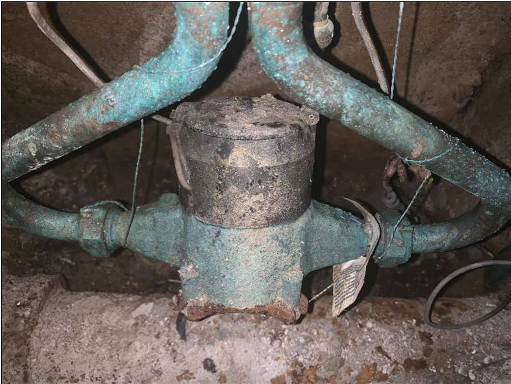
6.3 Item 2(Picture) Water meter.
