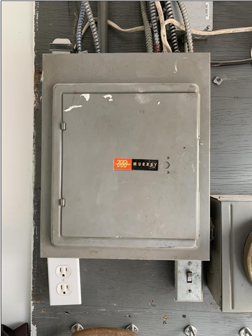
7.1 Item 2(Picture) Murray brand electrical panel.
