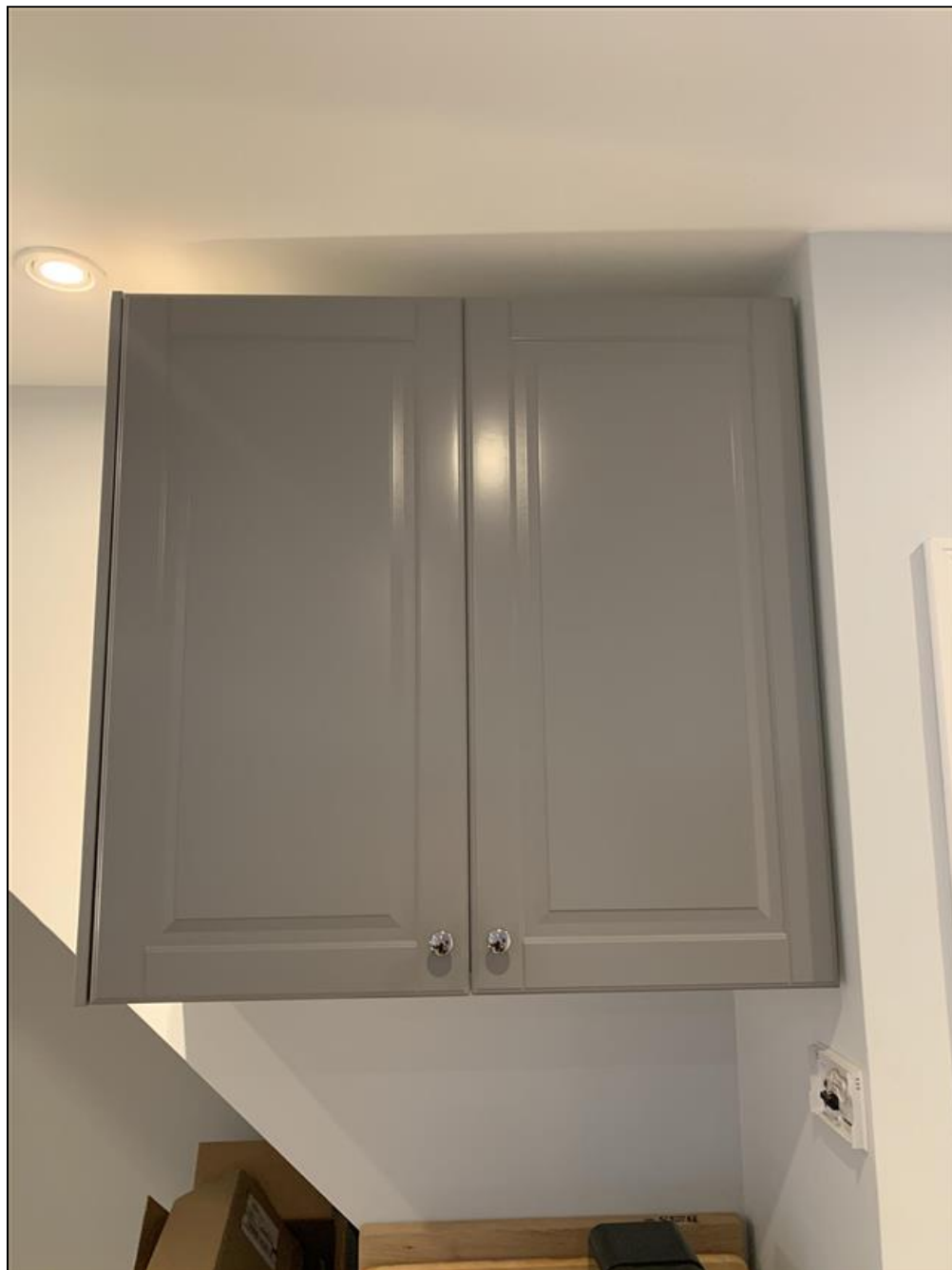
6.5 Item 1(Picture) Gas meter is located inside this cabinet near the first floor kitchen area.
