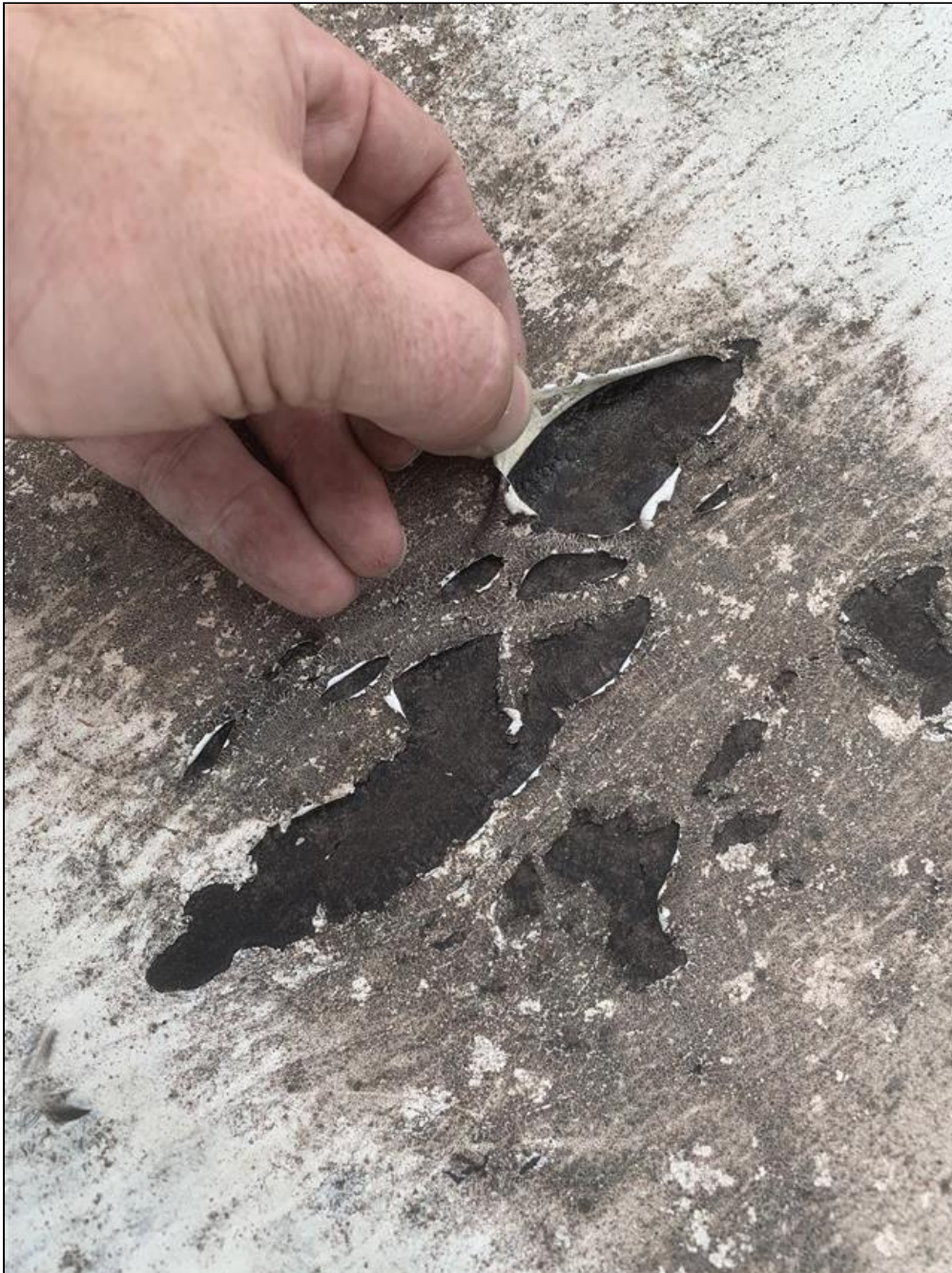
1.0 Item 4(Picture) Small spot near roof hatch where the silicone coating has worn away.
