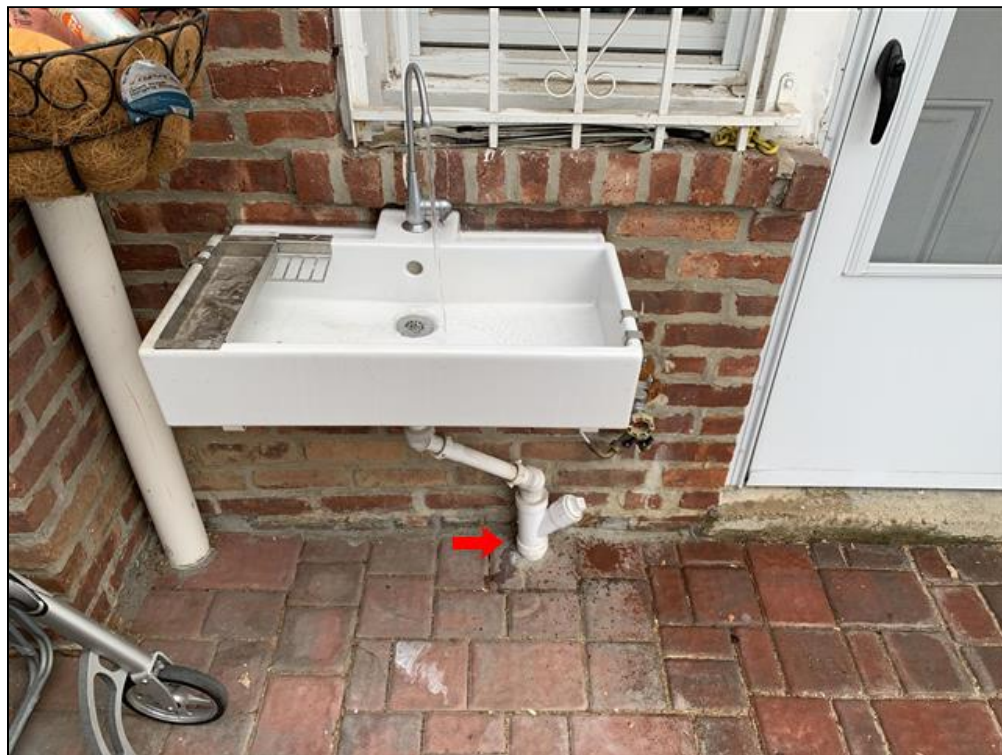
6.0 Item 4(Picture) Sink at back of home with leak location indicated.
