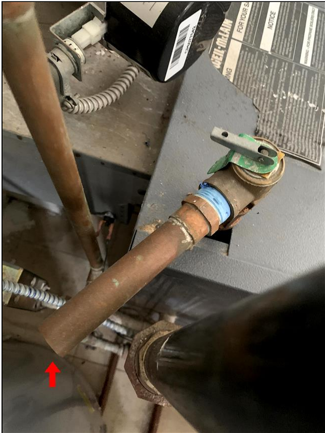
8.0 Item 6(Picture) TPR valve discharge pipe does not extend to 6 inches above the floor.
