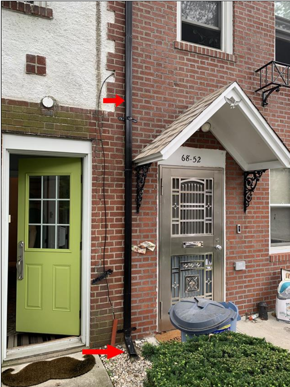
1.3 Item 6(Picture) Right-hand downspout terminates away from home but should extend further away from the foundation (ideally 8-10 ft but even 3-6 ft would be better).
