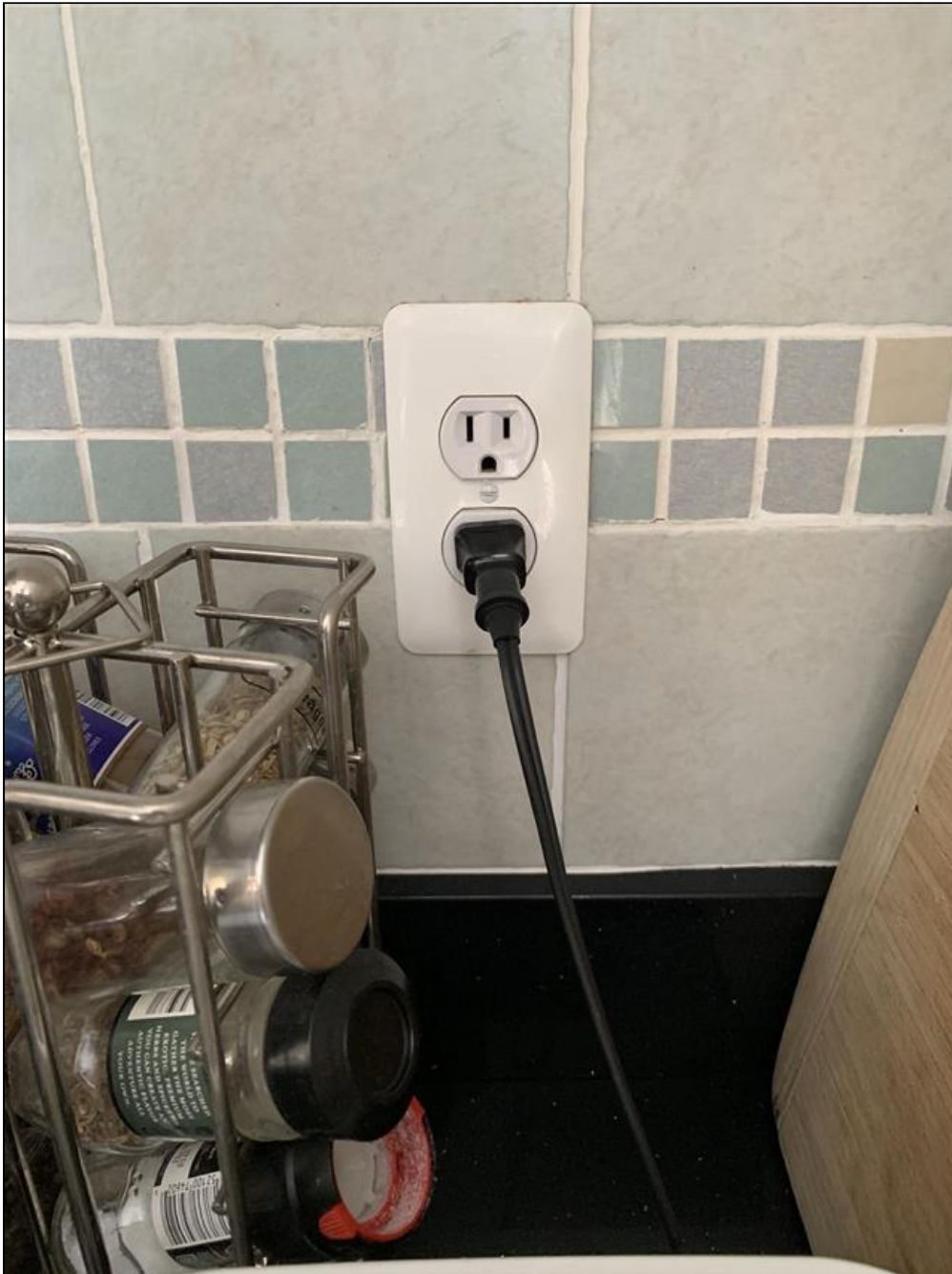
7.4 Item 3(Picture) Second floor kitchen counter: Electrical receptacles located within 6 feet of a plumbing fixture should be provided with GFCI protection.
