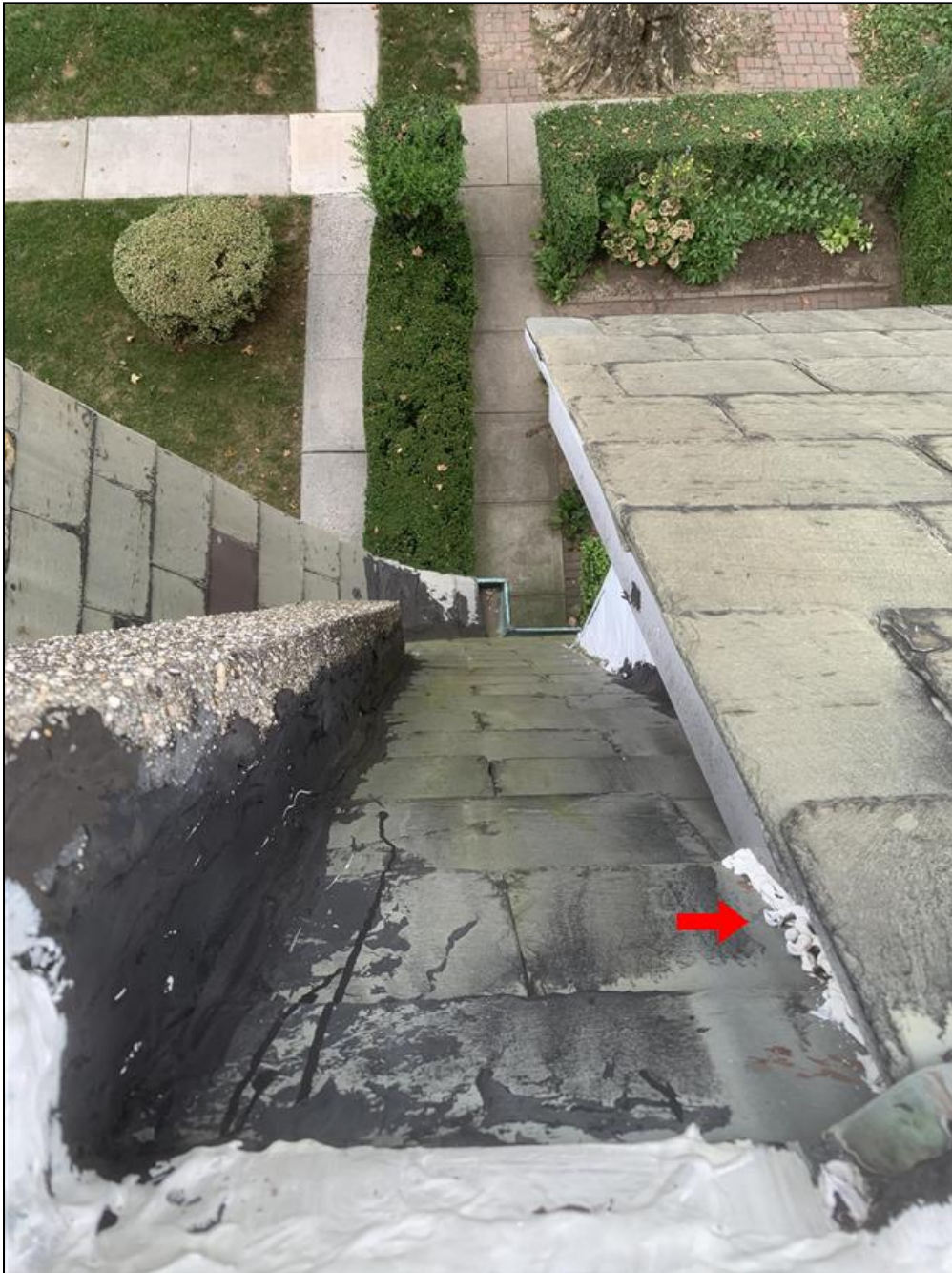
1.1 Item 4(Picture) Sealant at this location was applied very sloppy and does not appear to be doing much.
