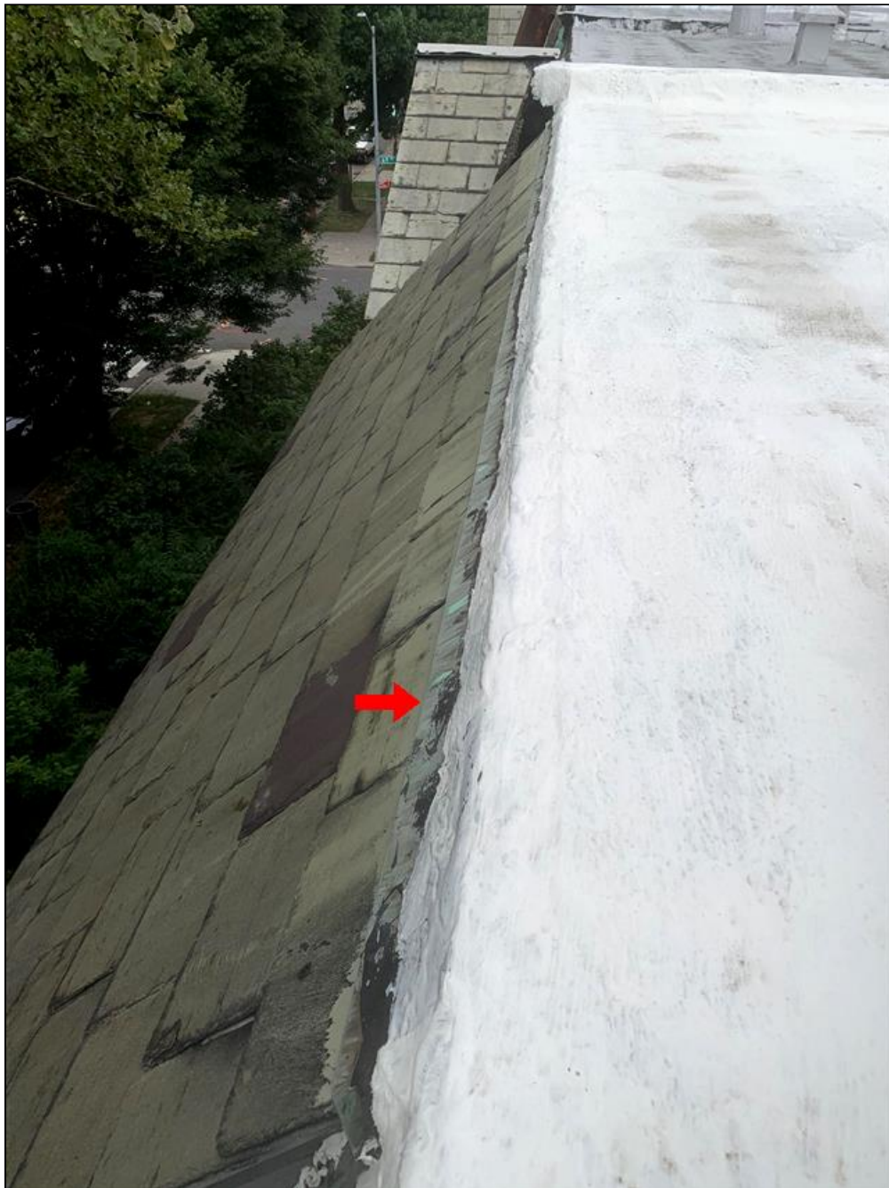
1.1 Item 2(Picture) At the front of the home metal flashing is installed above the slate roof (to keep water from getting below the slate) and then the roll roofing of the main room curls over the top edge of this flashing to keep water from getting behind the flashing.
