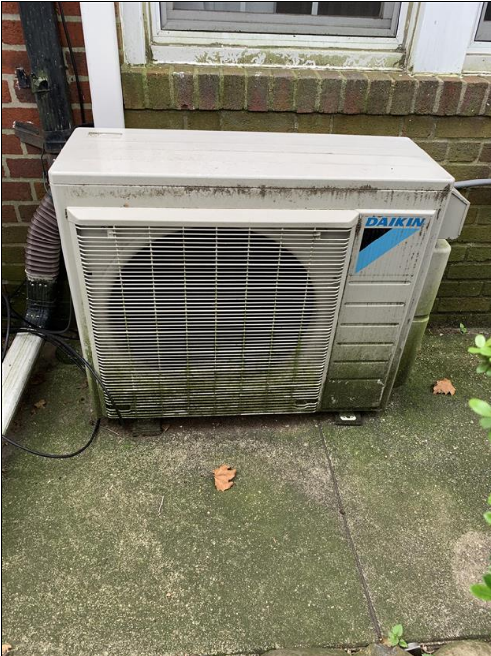
8.0 Item 2(Picture) Heat Pump at front of home.
