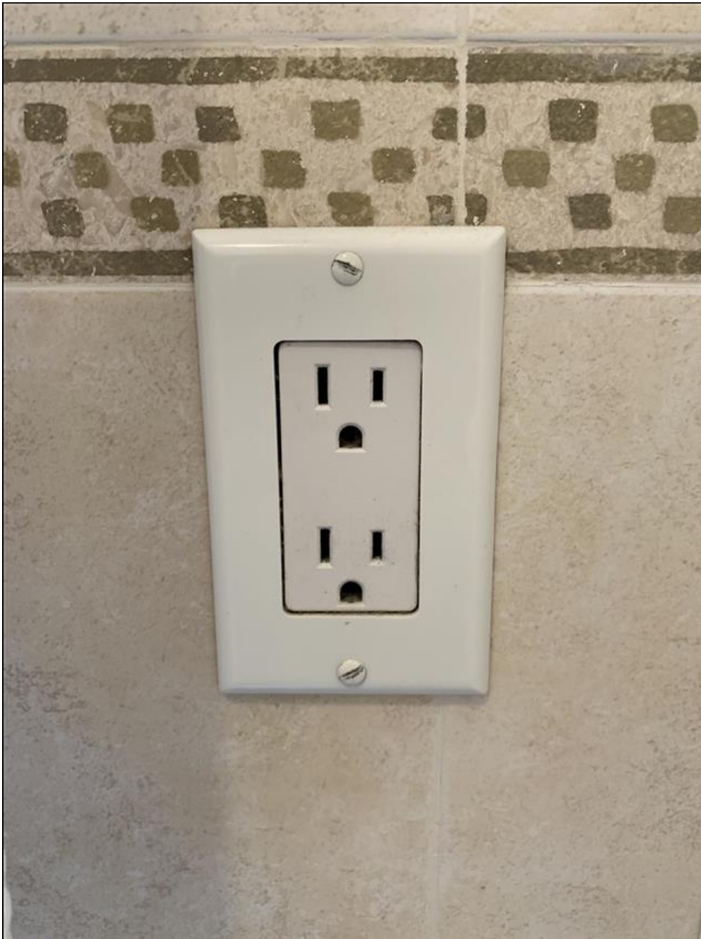
7.4 Item 5(Picture) Third floor bathroom: Electrical receptacles within 6 feet of a plumbing fixture should have GFCI protection for added safety.
