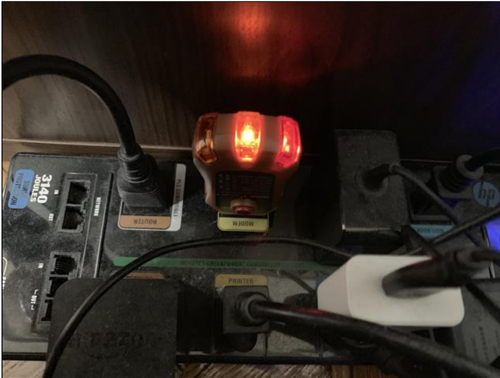
7.3 Item 10(Picture) Hot & neutral wires reversed.
