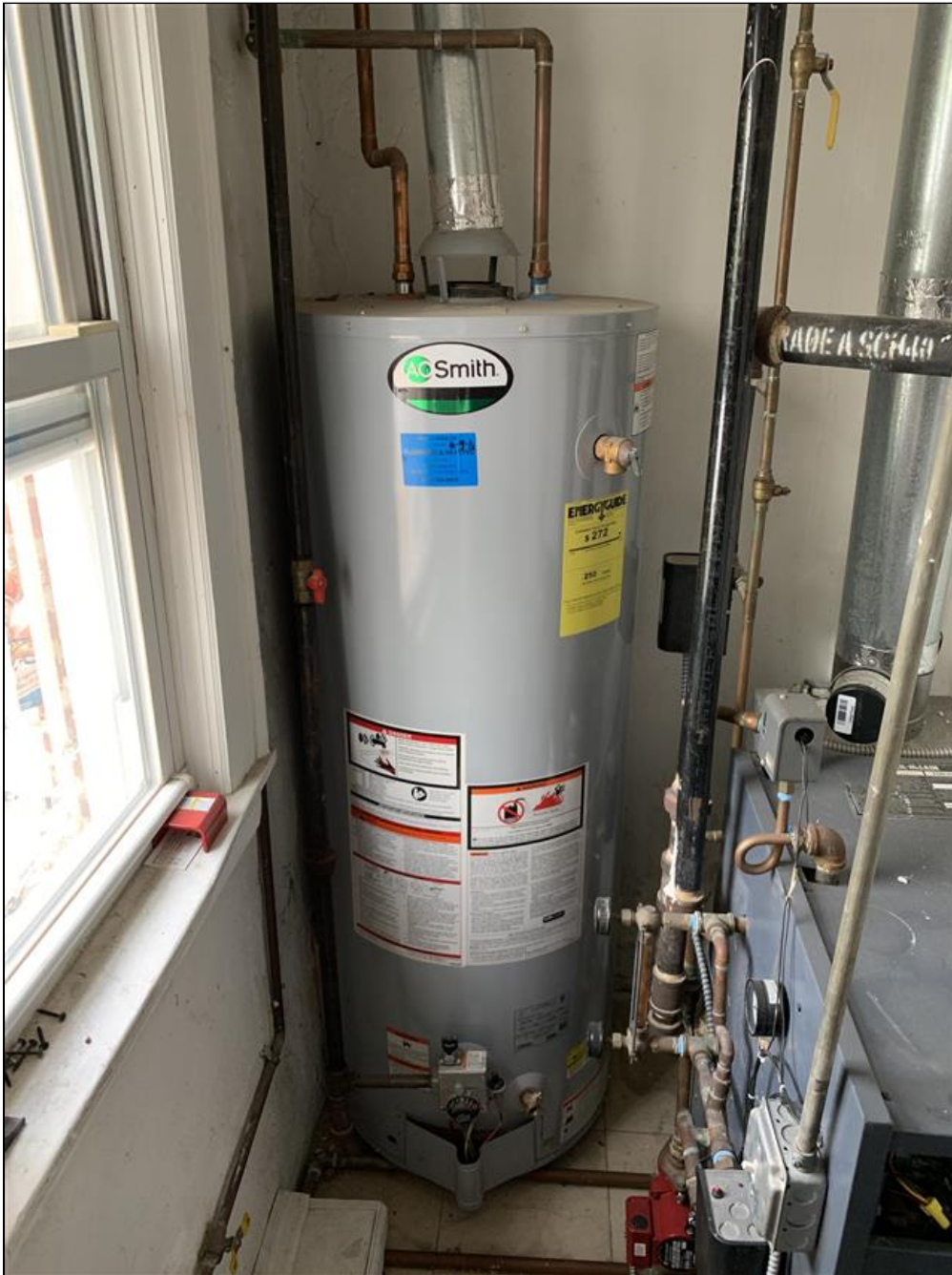
6.2 Item 1(Picture) A.O. Smith brand 50 gallon gas fired water heater.
