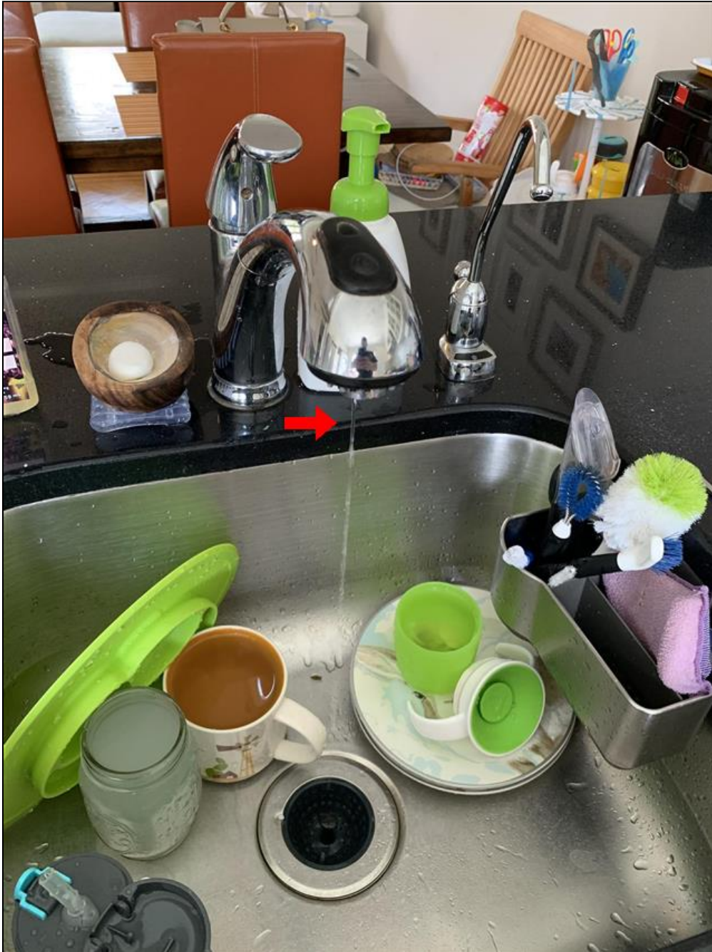
6.1 Item 1(Picture) Faucet still running when in off position.
