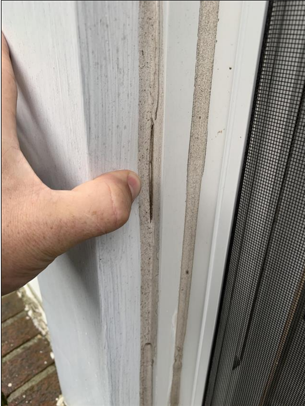
2.2 Item 3(Picture) Exterior window sealant has lost its seal.
