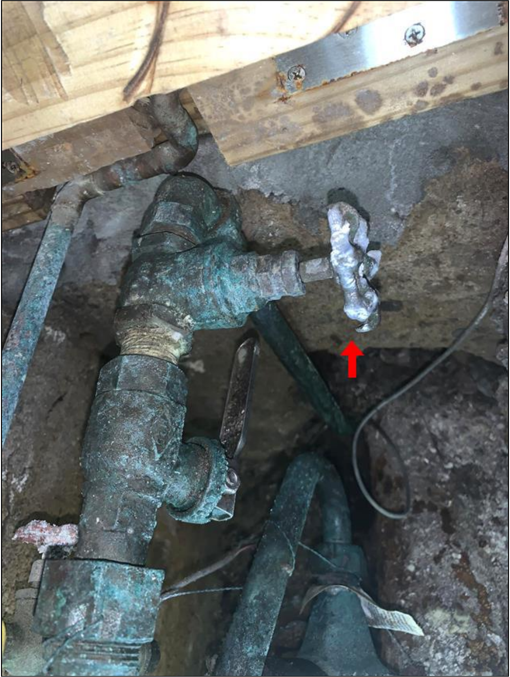
6.3 Item 3(Picture) Shutoff valve.
