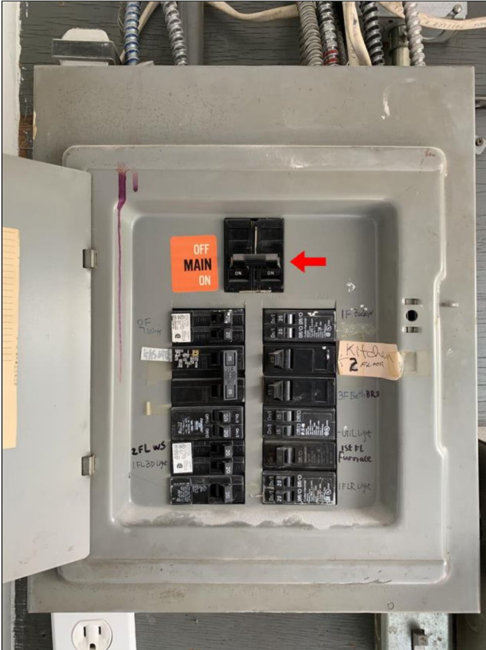
7.1 Item 1(Picture) Main overcurrent device.
