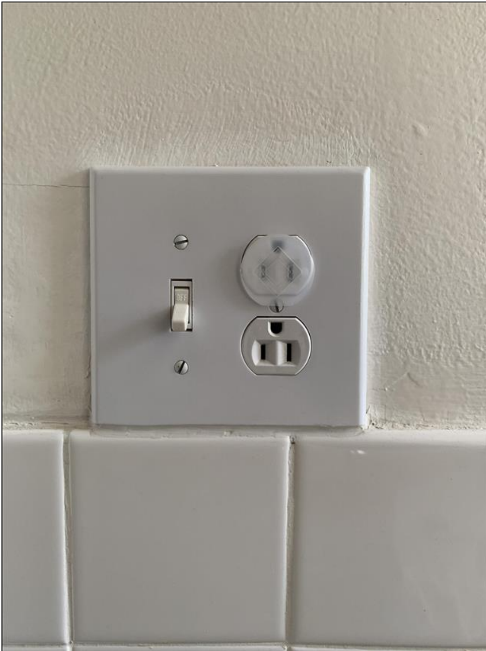
7.4 Item 4(Picture) Second floor bathroom: Electrical receptacles within 6 feet of a plumbing fixture should have GFCI protection for added safety.
