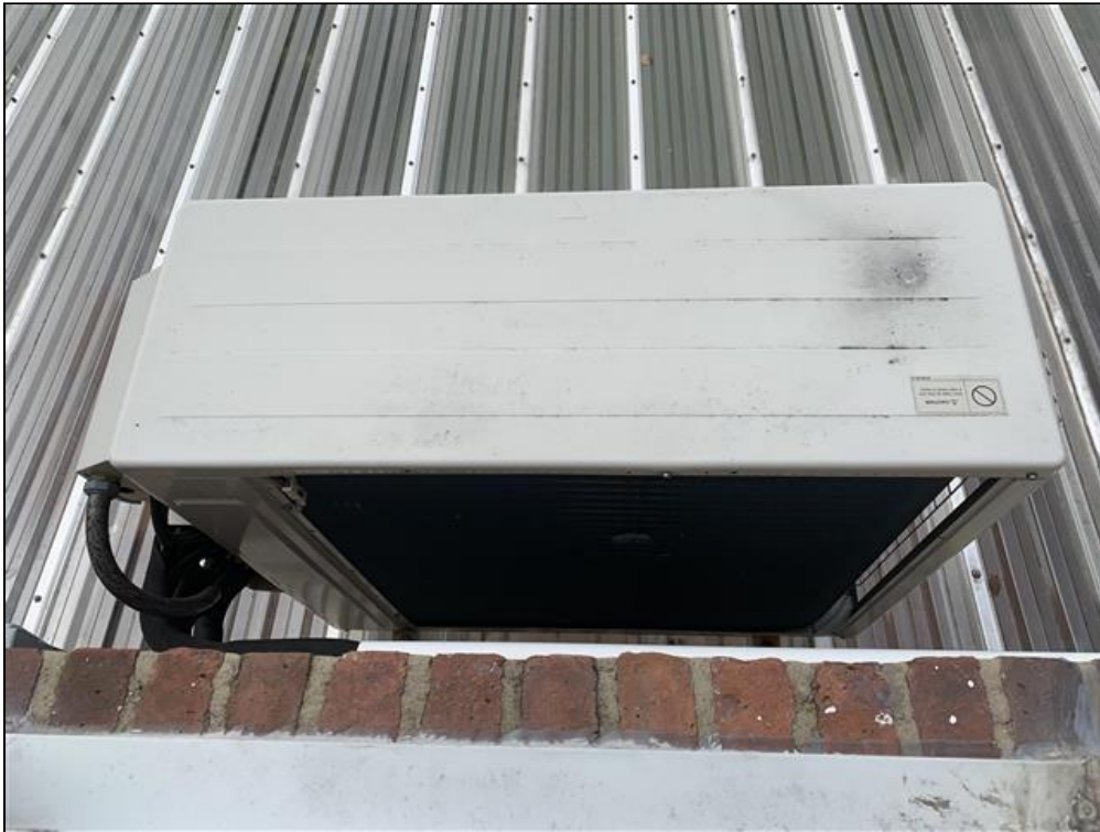
8.8 Item 2(Picture) Heat Pump mounted outside second floor kitchen window.
