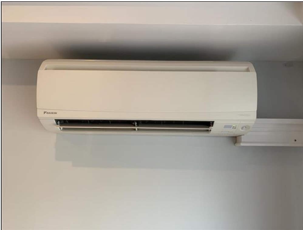
8.8 Item 3(Picture) Example photo of indoor fan coil units (6 total).
