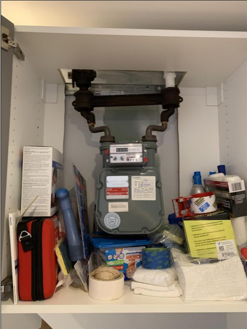
6.5 Item 2(Picture) Gas meter.
