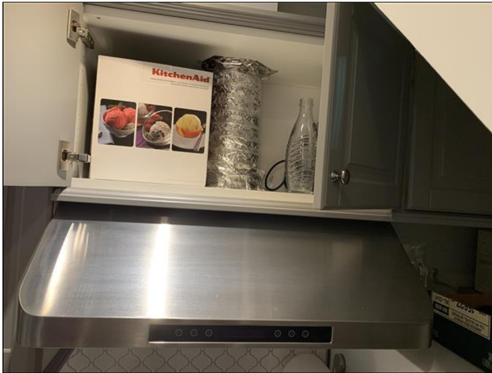
10.1 Item 1(Picture) Range hood on first floor.
