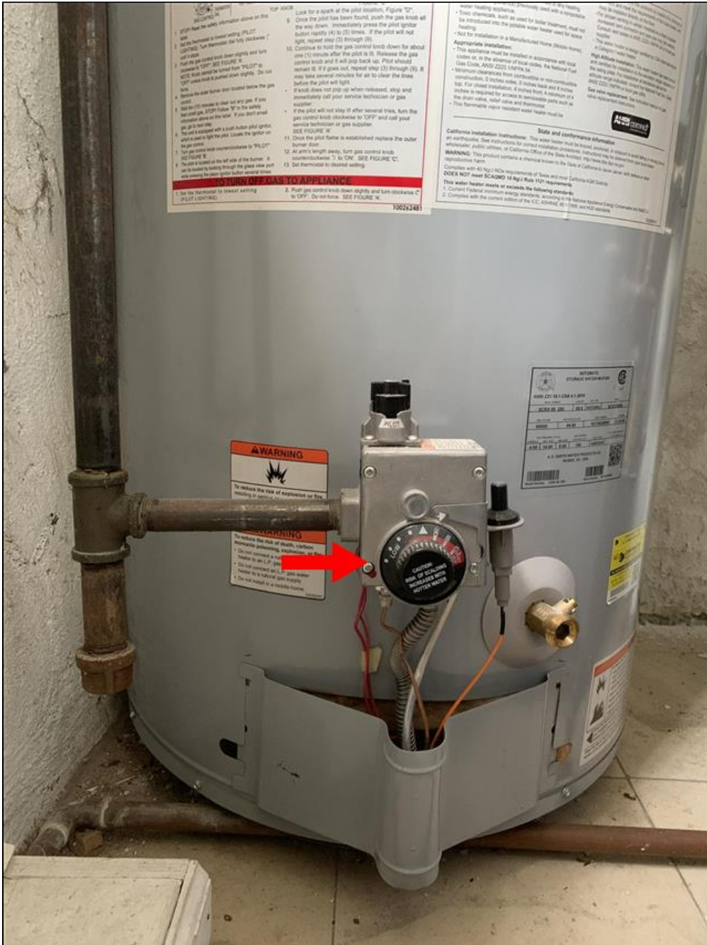
6.2 Item 4(Picture) Hot water temperatures can be controlled here.
