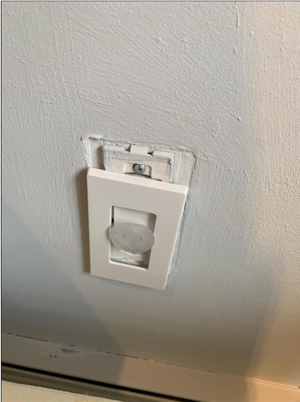
7.3 Item 1(Picture) Face plate is loose and falling off.
