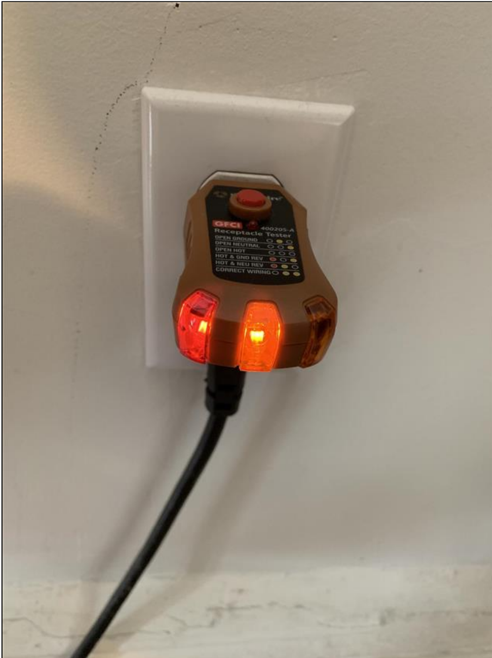
7.3 Item 6(Picture) Hot & neutral wires reversed.
