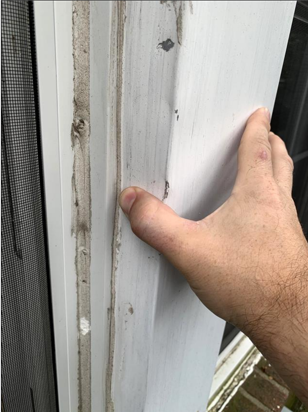
2.2 Item 1(Picture) Exterior window sealant has lost its seal.
