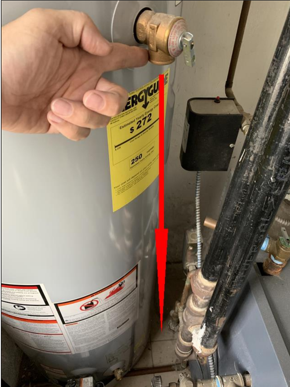
6.2 Item 5(Picture) A TPR valve extension pipe should be installed here for safety.
