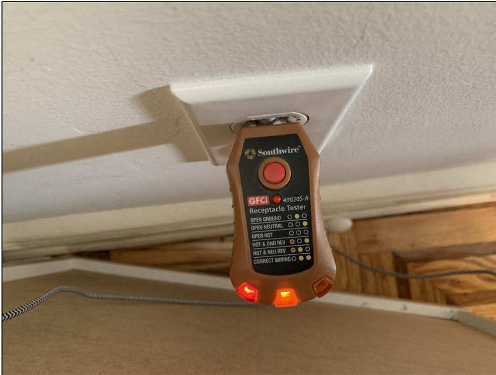
7.3 Item 7(Picture) Hot & neutral wires reversed.
