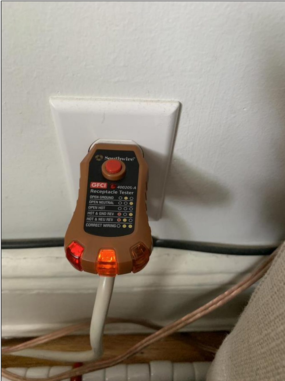
7.3 Item 8(Picture) Hot & neutral wires reversed.
