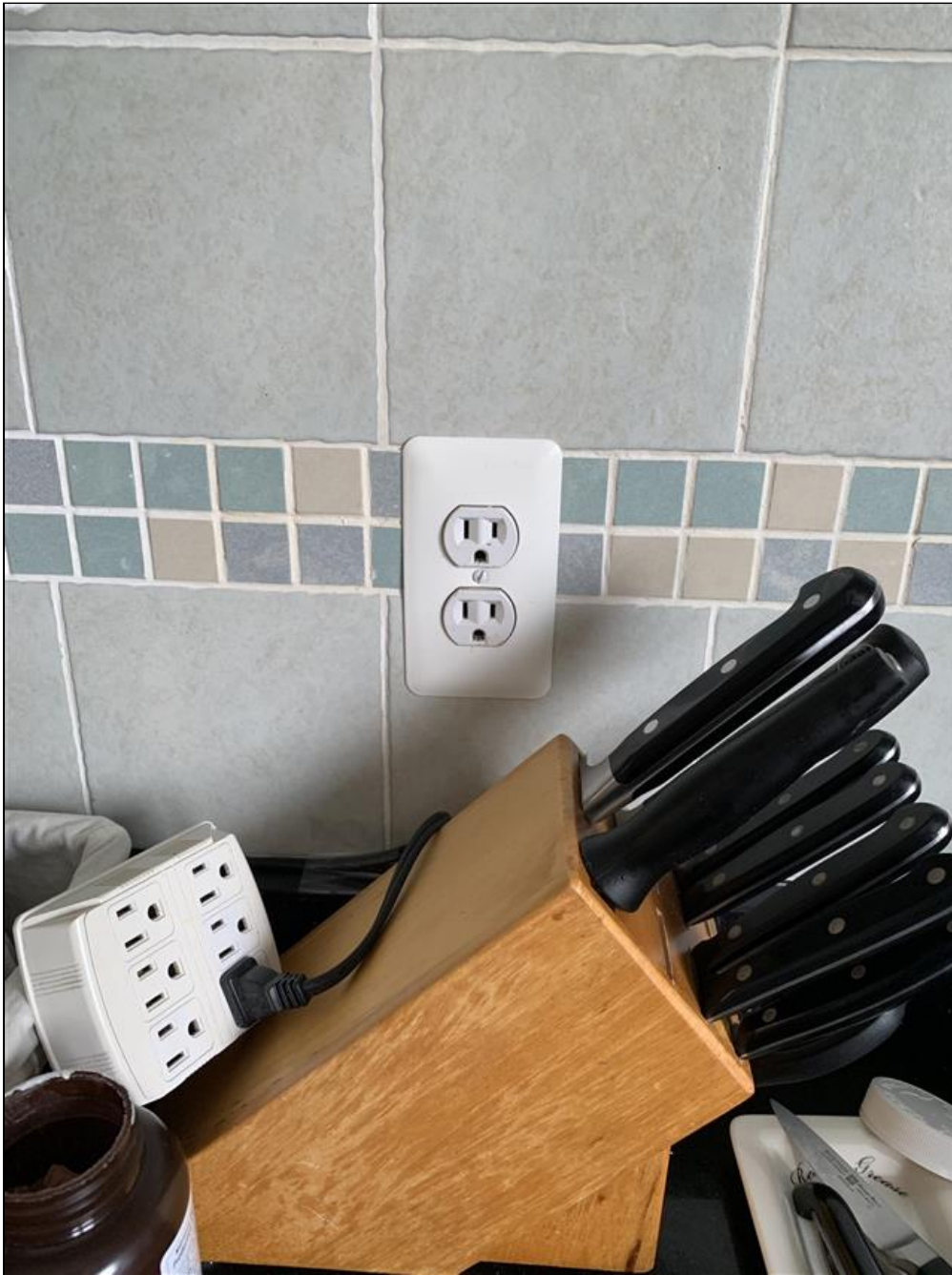
7.4 Item 2(Picture) Second floor kitchen counter: Electrical receptacles located within 6 feet of a plumbing fixture should be provided with GFCI protection.
