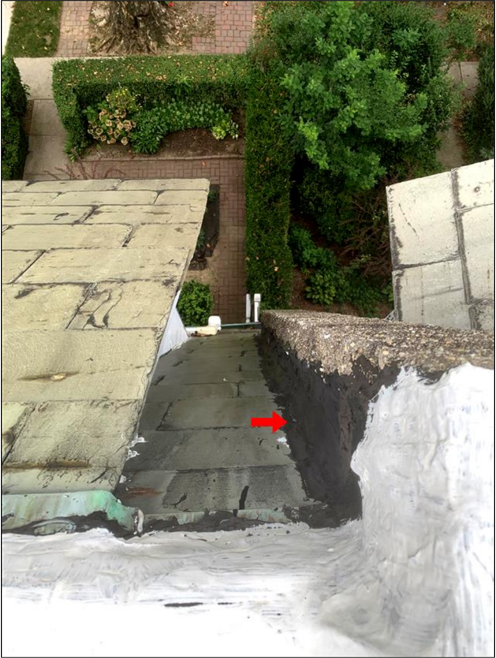
1.1 Item 5(Picture) Flashing cement used here appears to be holding its seal but will eventually need maintenance.
