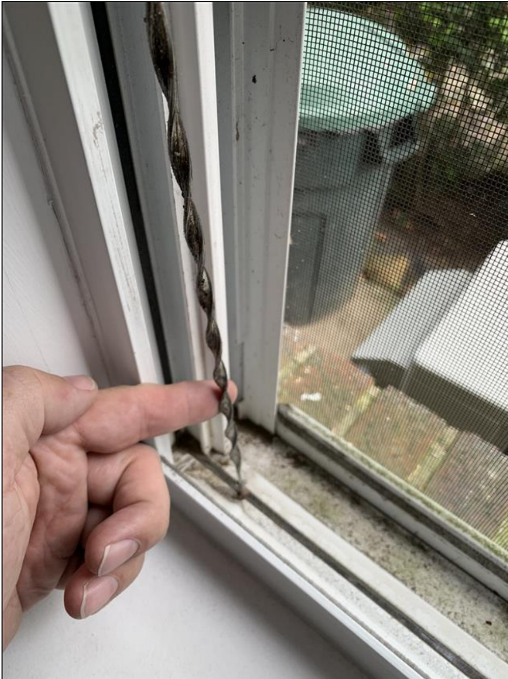
4.7 Item 1(Picture) One of the window channel balances was found to be disconnected or broken in the first floor bedroom (right most window).
