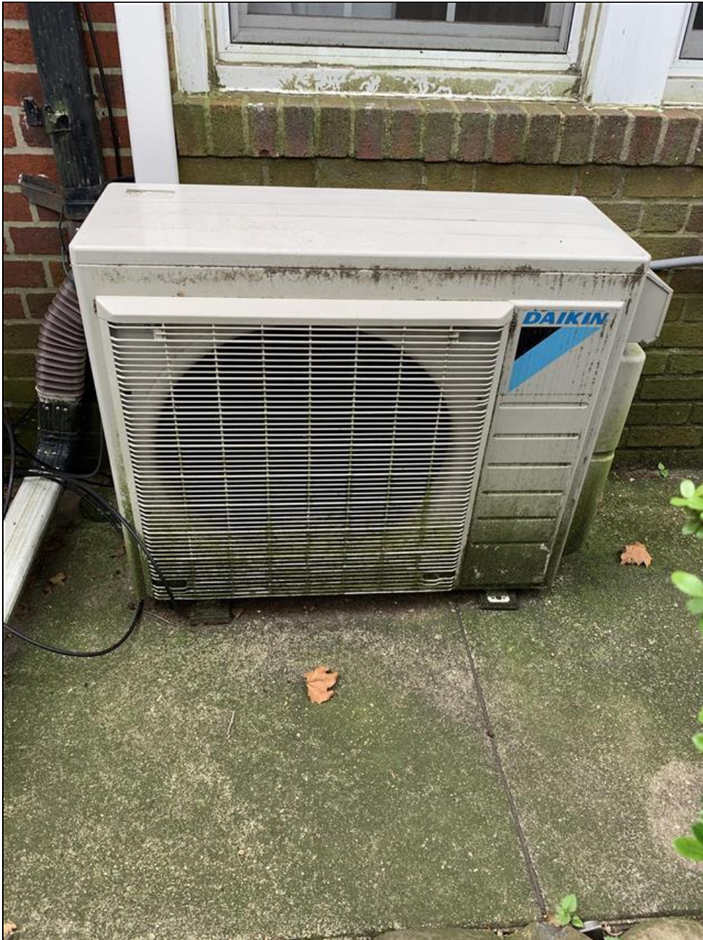
8.8 Item 1(Picture) Heat Pump at front of home.
