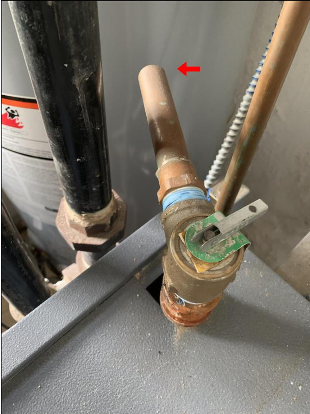
8.0 Item 5(Picture) TPR valve discharge pipe does not extend to 6 inches above the floor.
