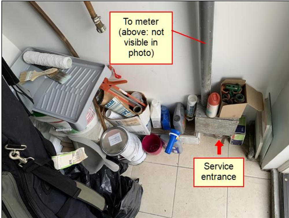
7.0 Item 1(Picture) The main service entrance conductors enter the utility room located at the rear of the home from below ground.
