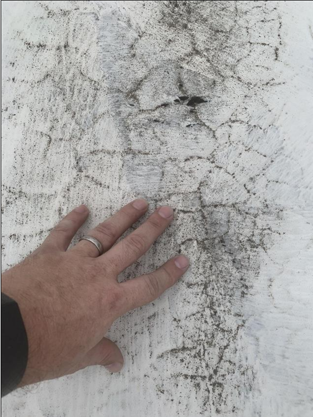
1.0 Item 3(Picture) A cracking pattern below the silicone coating was noted in some locations.
