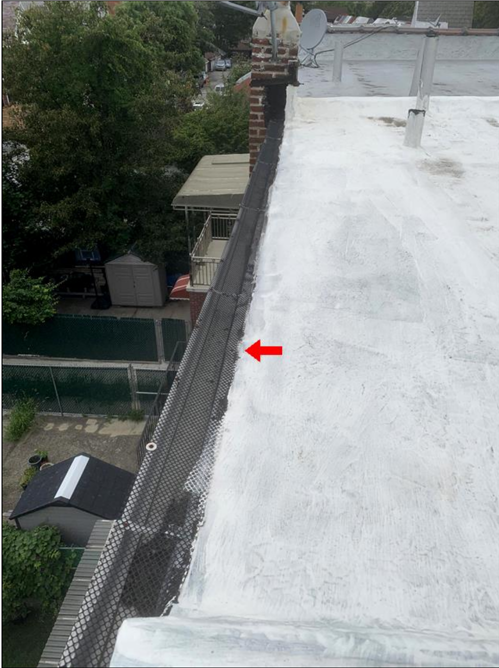
1.1 Item 1(Picture) At the rear of the home the roof cladding curls over the edge and acts as edge flashing.
