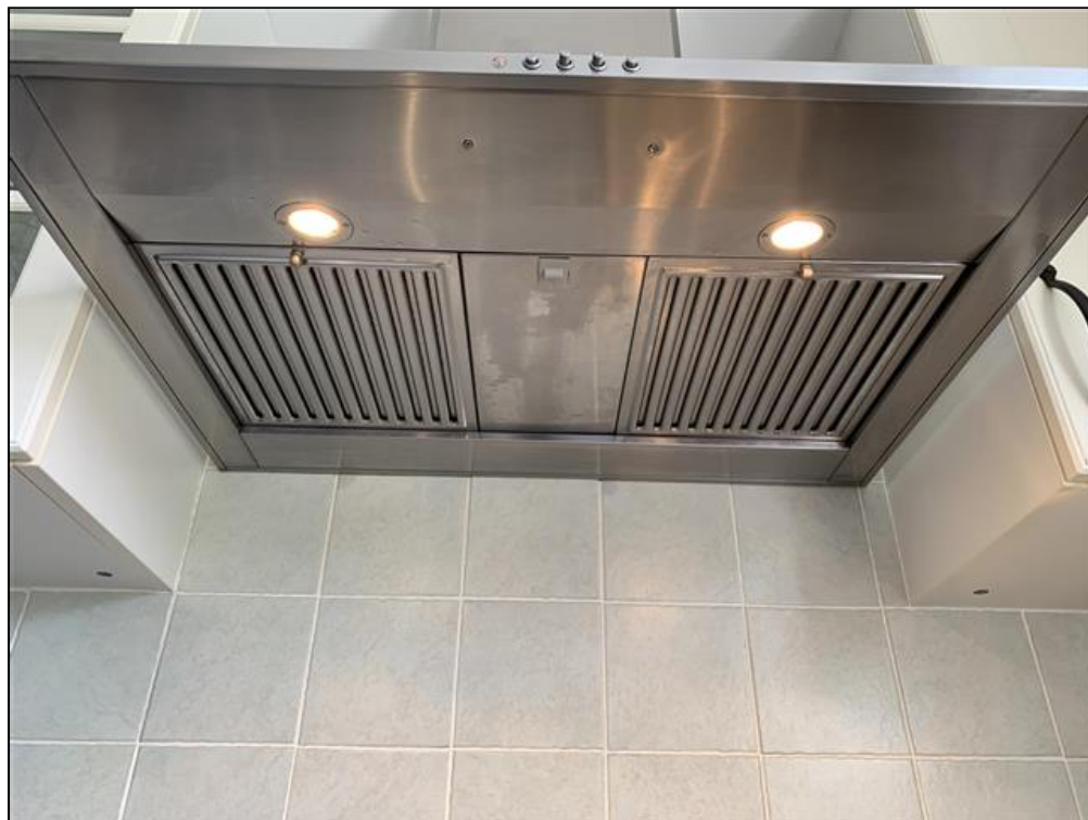
10.1 Item 4(Picture) Range hood on second floor.
