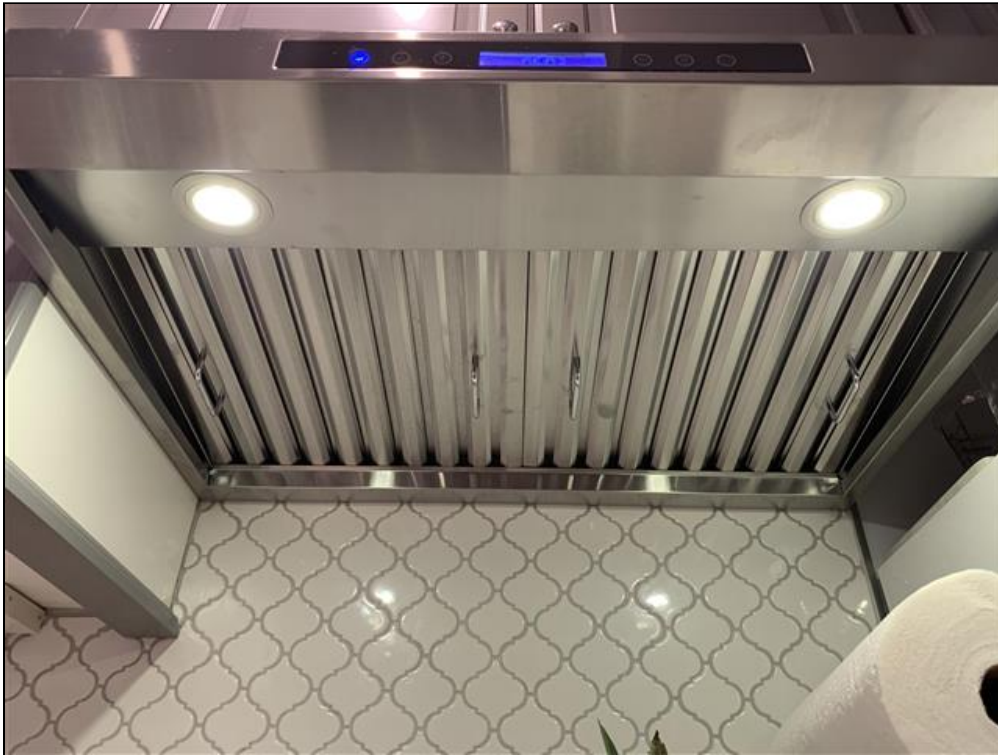
10.1 Item 2(Picture) Range hood on first floor.
