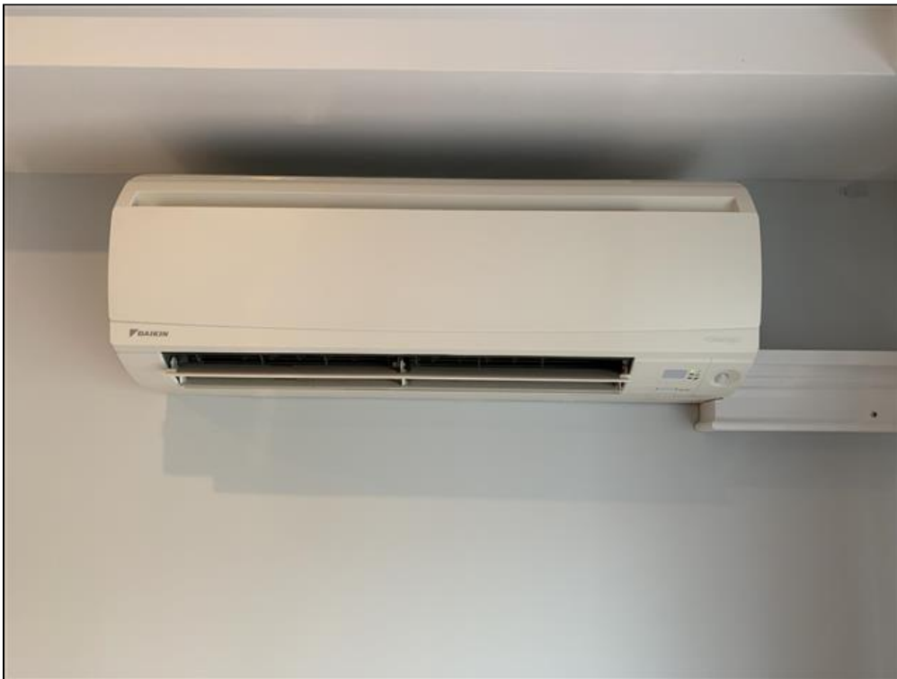
8.0 Item 4(Picture) Example photo of indoor fan coil units (6 total).
