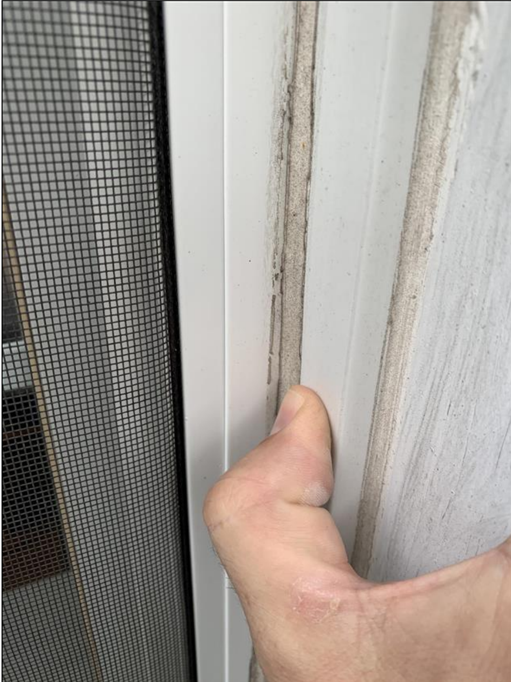
2.2 Item 4(Picture) Exterior window sealant has lost its seal.
