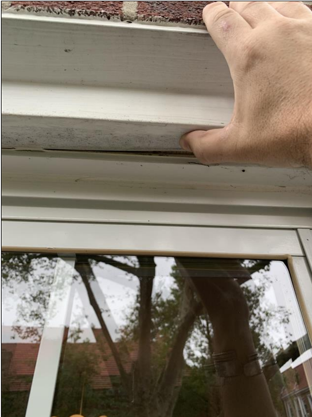
2.2 Item 2(Picture) Exterior window sealant has lost its seal.
